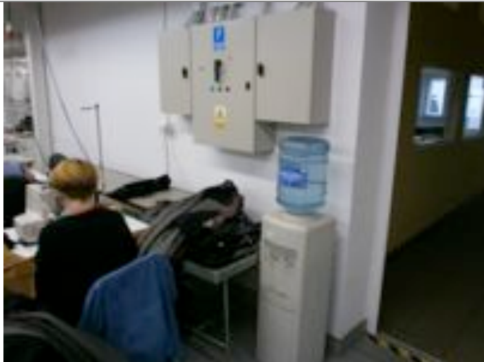
Cluster N° 8.3 Electrical fuse box obstructed and has no isolation
